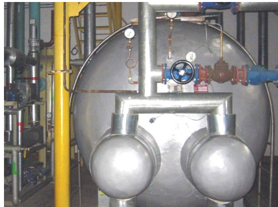
Previous Storage Water Heater
